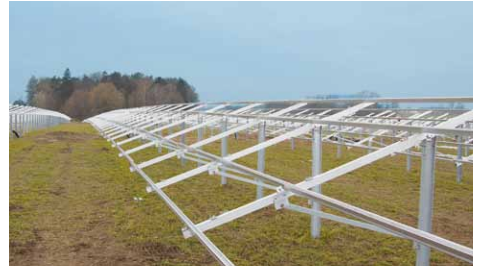
Nierpars | Germany System: 3,942 MW | T-Rack System
